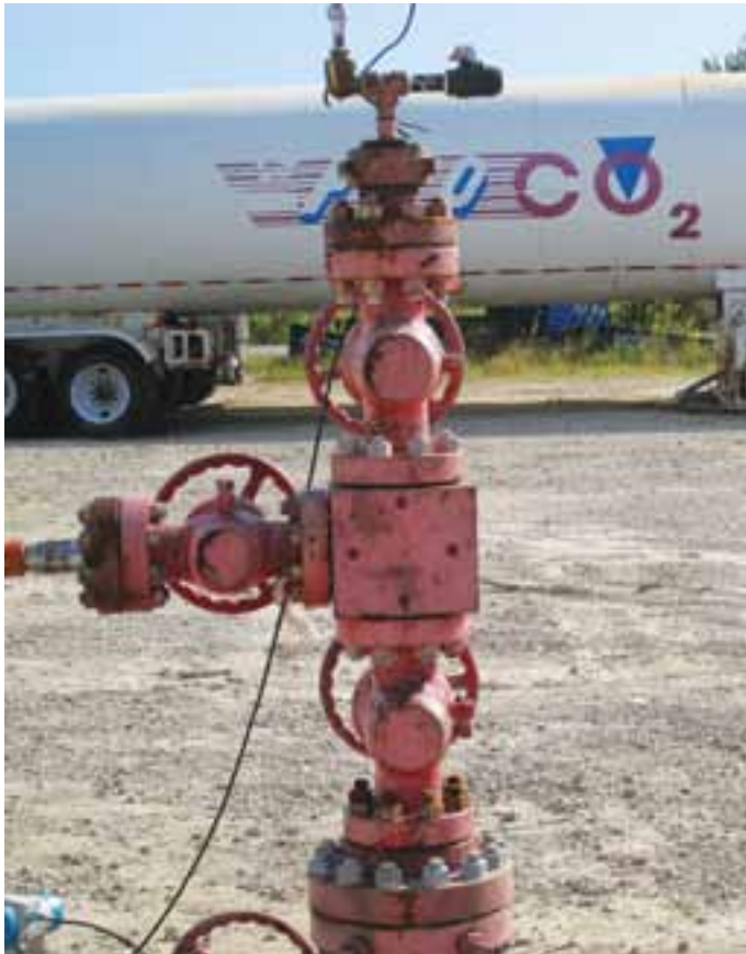
An injection well marks the site of a carbon sequestration research project at Mississippi Power's Plant Daniel, where 3,000 metric tons of CO 2 were injected into a deep saline rock formation below ground.
