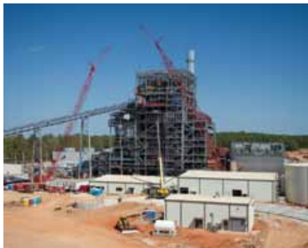
Construction of the 100-megawatt biomass plant being built by Southern Power in Sacul, Texas, continues.
